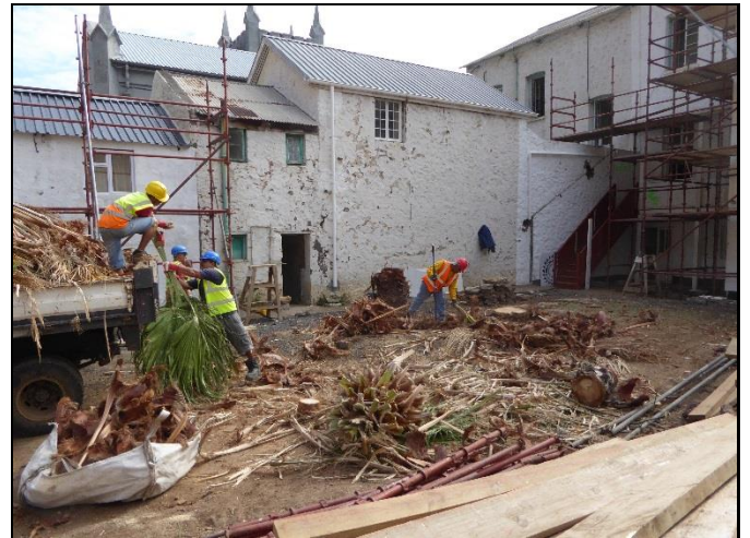
Clearance underway at the rear of site with the church in the background
